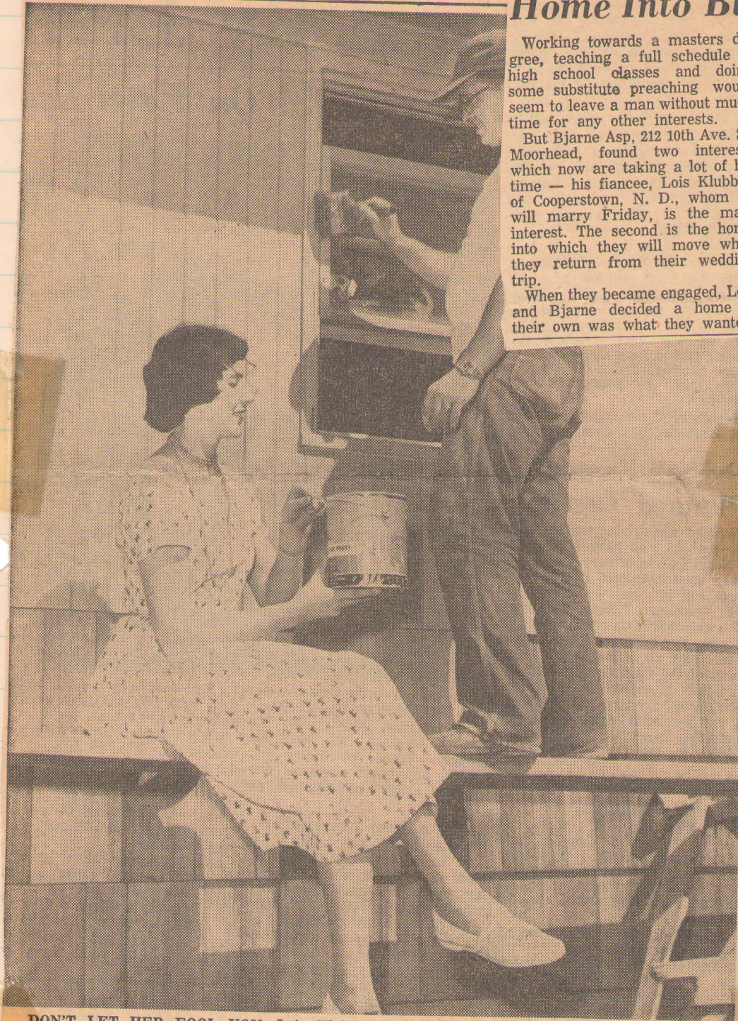
DON'T LET HER FOOL YOU, Lois Klubben has done more than pose gracefully with a paint pail, during the construction of the house she and her fiance, Bjarne Asp will live in following their marriage Friday. (Fargo Forum Photo)
